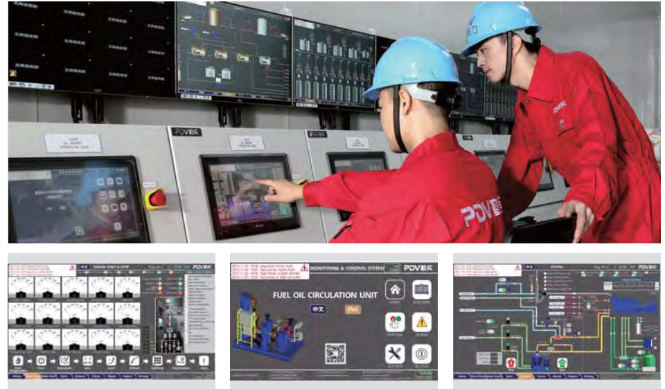
Electrical Control System (SCADA)
