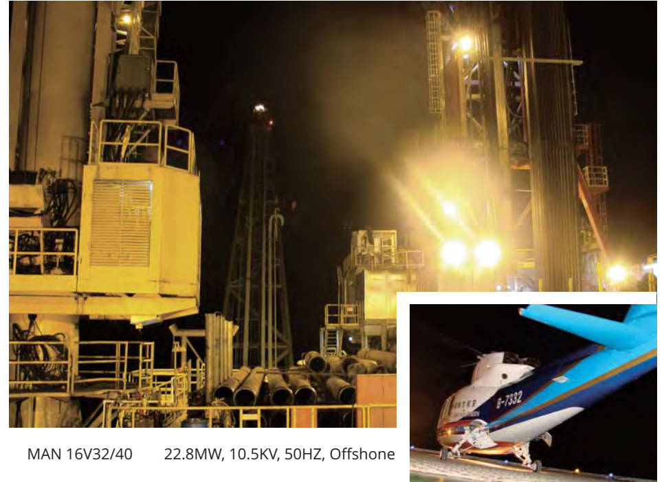
LF14-4 Crude Oil Engine Generator Sets And Auxiliary System In China Offshore
