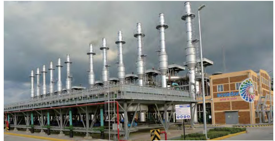
Pielstick 12PC2-6B 100MW, 13.8KV, 60HZ, Base Load, to the National Grid
